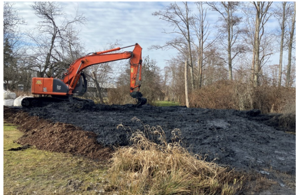
The same area as above photo once the Cattail had been dug out to reclaim the clogged channel and the organic matter had been consolidated and buried in the native silts. Photo: Kathleen Fry
